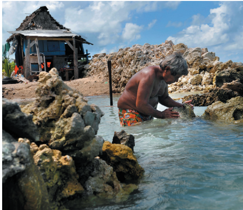
A man rebuilds the sea wall that protects his home on South Tarawa.
