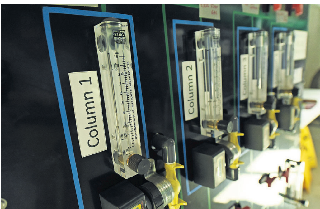
ABOVE: Granular activated carbon (GAC) filter systems, such as the one seen here at the CFPWA Sweeney Water Treatment Plant in North Carolina, is one method water systems are using to treat PFAS and other chemicals. [STARNEWS FILE]
